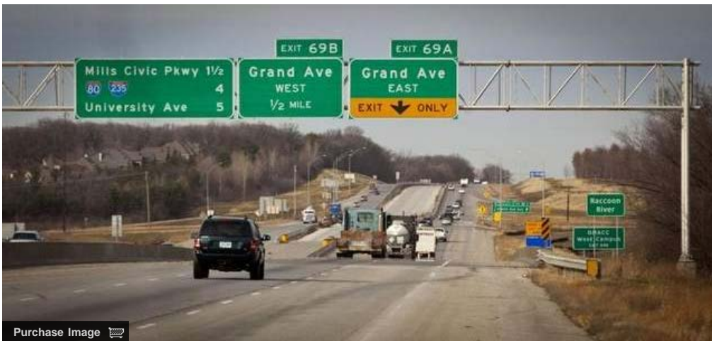
Construction of extra lanes along I-35 south of the west mixmaster Nov. 26 in West Des Moines. / Rodney White/The Register
